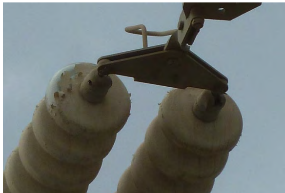
Figure 10: Example of poor adherence resulting from poor application on site and lack of cleanliness
