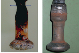
Corroded pin without zinc sleeve
