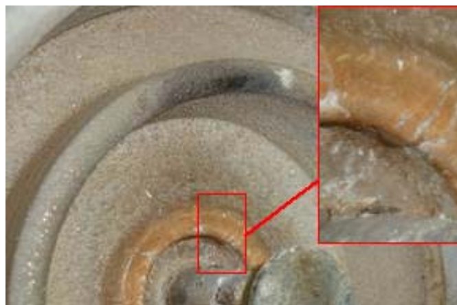
Figure 5. Heavily polluted insulator after 7 ½ years showing very light surface erosion on the HV end unit: Brindisi 380 kV line, USCD: 38 mm/kV. Inset: Close-up of the first under-rib.
