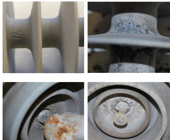
Figure 4: Comparative ageing pattern between a silicone coated composite insulator and an equivalent string of silicone coated toughened glass insulators.
