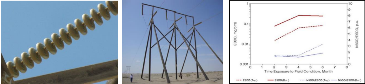
Figure 15: Under-coating toughened glass insulators in Peru (Chiclayo area)
