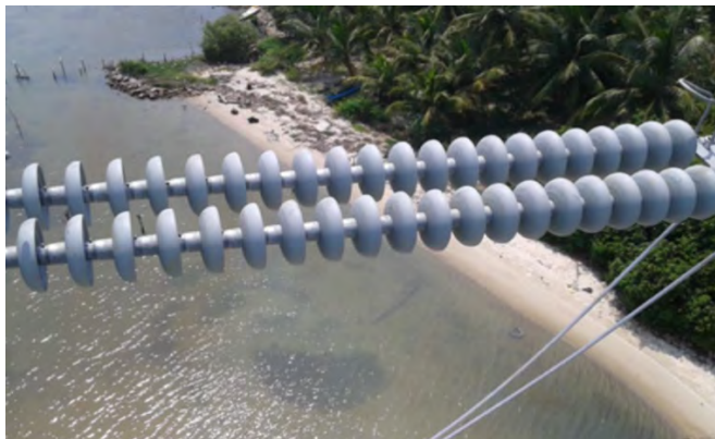
Figure 3: Silicone coated glass insulators (220kV transmission line Sri Lanka USCD = 31,5mm/kV)
