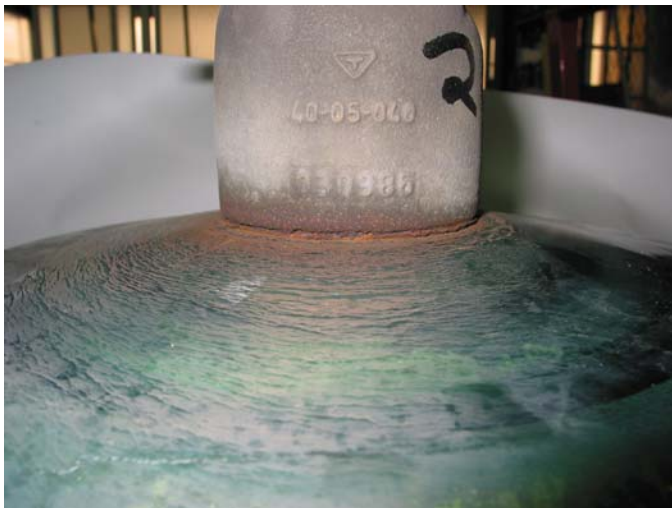
Figure16 : corrosion at the base of the cap on a few units
