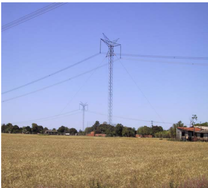
Figure12: Itaipu I and Itaipu II +/-600 KV DC equipped with SEDIVER toughened glass insulators
