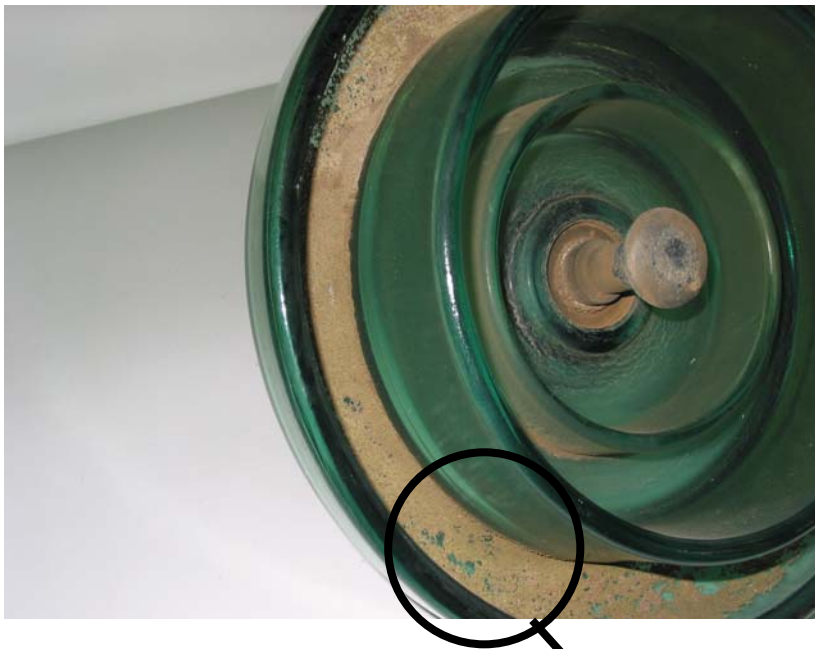
Figure 13: pollution concentration in external section of the bottom of the insulator outside the large rib while the rest of the insulator remains clean
