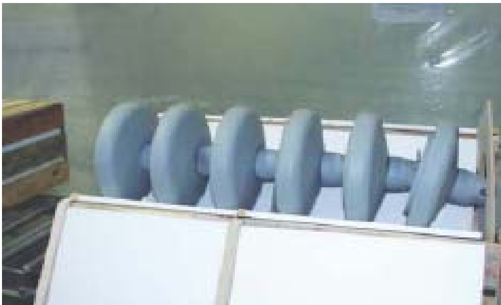
inside protection of a coated insulator box
