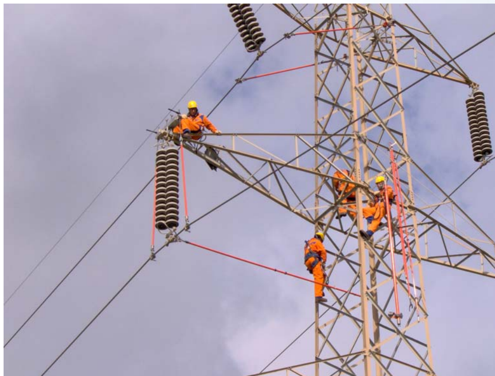
Installation of coated insulators on a 220 kV live line in Sicily, South of Italy
