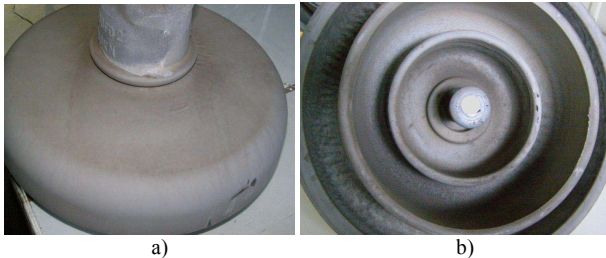
Fig. 2. Visual inspection: a) insulator #12 top surface with a lateral scrape; b) insulator #1 bottom surface with dirt under ribs and without interesting signs of degradation.
