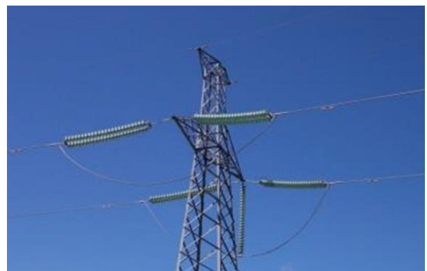
Figure 8 silicone coated toughened glass insulators installed in Italy on the Terna 200kV dc line.
