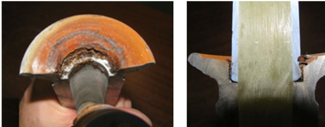
Figure 9. Corrosion and degradation of the seal of a polymer insulator at the triple point resulting in moisture ingress and major risk of failure. (removed from service after a decade)
