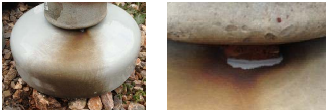
Figure 8. Damaged porcelain insulator resulting from the lack of zinc collar and excessive gap.
