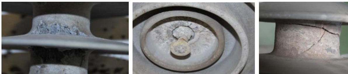
Figure 8: Left and centre: comparison of ageing of a silicone polymer and silicone coated glass in Koeberg test station, South Africa, with strings having the same leakage distance tested in parallel. Right: compromised integrity of a polymer insulator that is still hydrophobic but has deep cracks after 10 years in coastal pollution.
