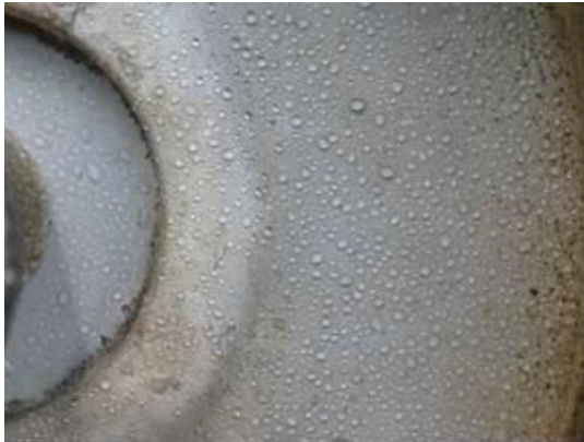
Figure 7: Water repellent hydrophobic property of silicone even over a polluted surface (silicone coated glass insulator after more than 10 years in a very heavy polluted environment).
