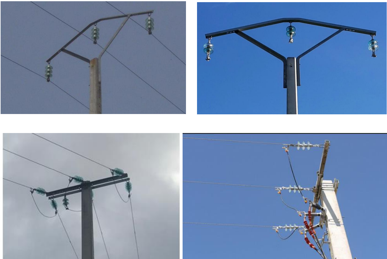
Figure 22 : examples of resilient distribution lines using concrete poles and toughened glass insulators in suspension and tension.
