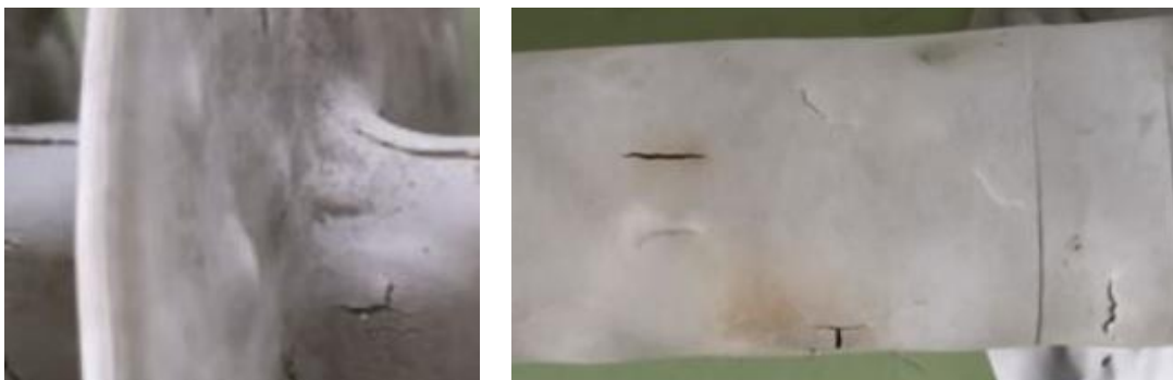
Figure 21: Cracks in silicone housing left after being subjected to heat for a few hours
