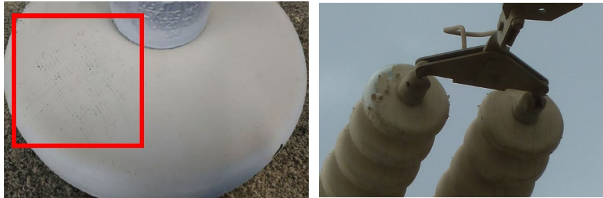
Figure 6: Left: adherence scratch test. Right: Bad application with adherence problem [9].
