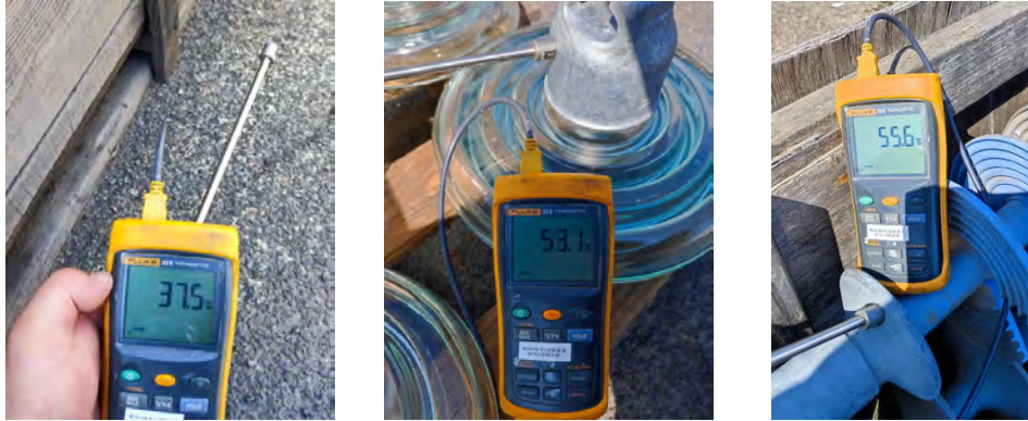
Figure 2 : Temperature gap between air temperature and contact on insulator fittings
