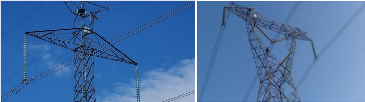
Figure 5: Examples of Sediver Smart insulators field installations (Left: 500kVDC, Right 500kVAC) for real time leakage current monitoring and diagnostics.
